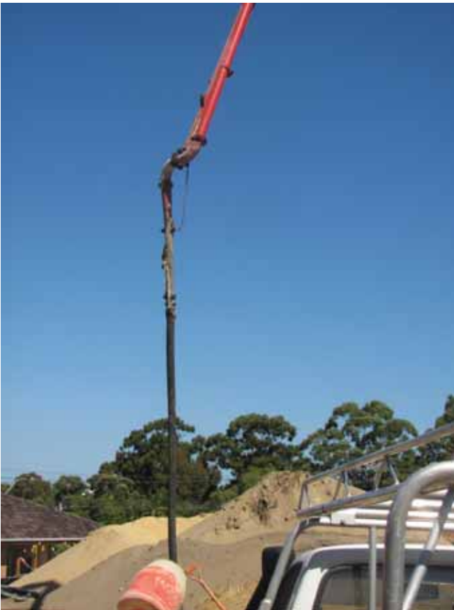
Delivery hose secured by safety chain
