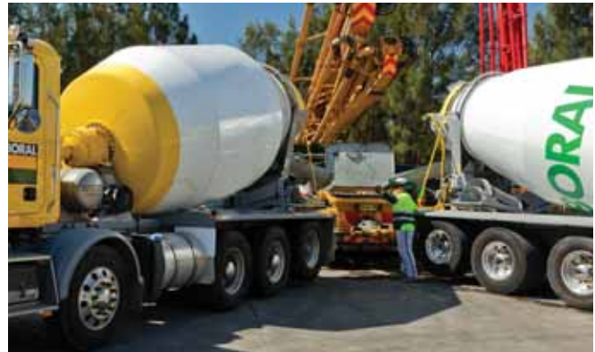
A truck spotter, in correct PPE, reversing a concrete agitator onto the concrete pump. Two trucks on the feed with over 600mm clearance.
