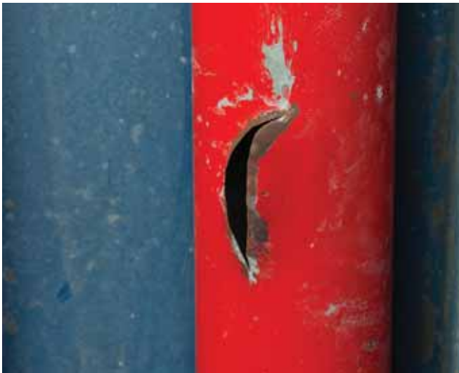
A damaged concrete pipeline
