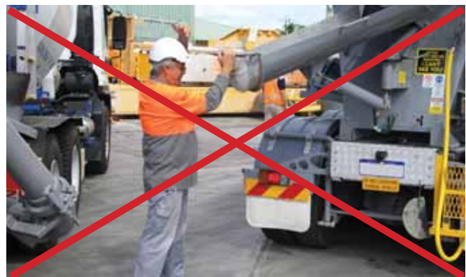
Unsafe spotter without appropriate PPE and position adjusting concrete chute while truck is reversing
