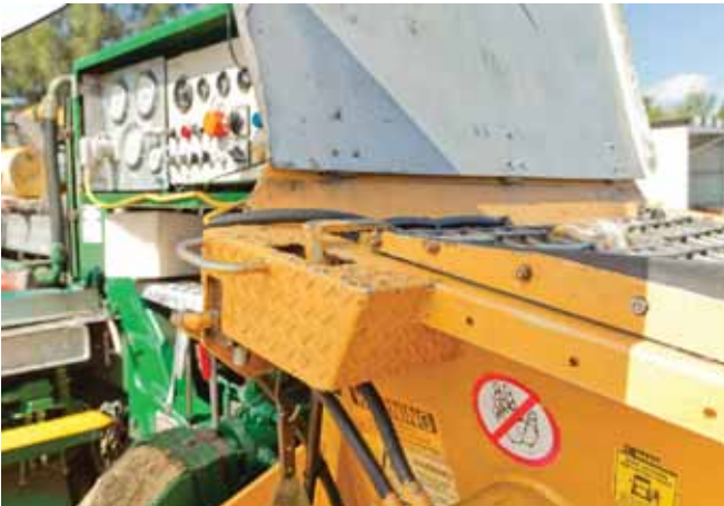
Interlocking mechanism which shuts down the pump if the grate is lifted
